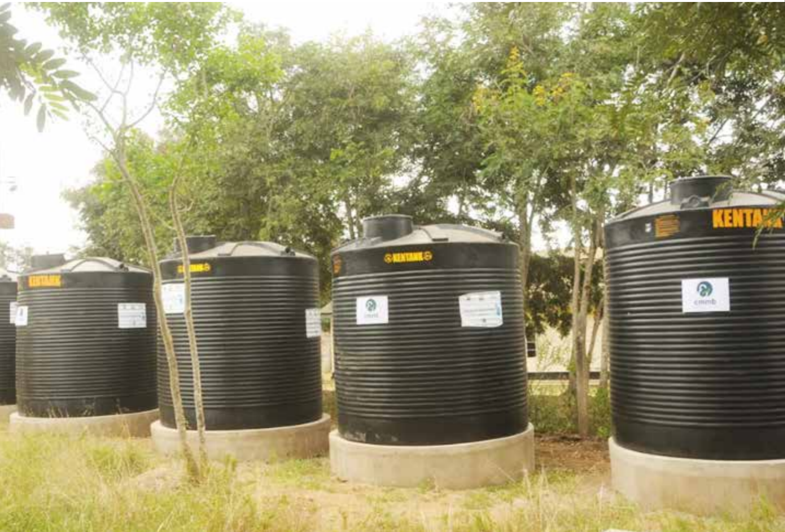
Rainwater harvesting tank and gutter system installed by CMMB at a health facility in Kitui County
